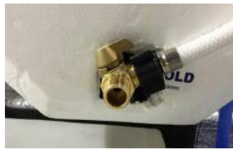
Figure 2 Water Heater Valve in Bypass Position
